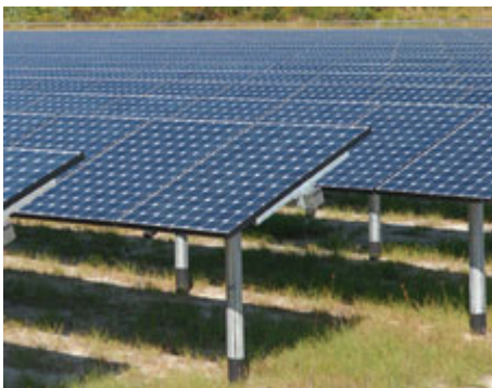
More than 3,300 solar panels have been erected on a vacant five acres at KSC in Florida
